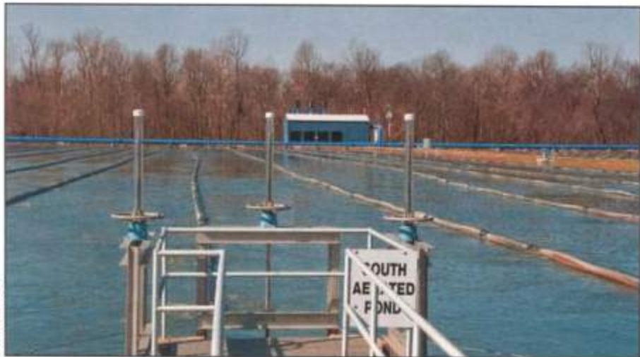
Floating-baffle curtains, constructed of reinforced rubber, partition the plant's aerated lagoons into complete-mix and partial-mix sections to increase treatment efficiency.
