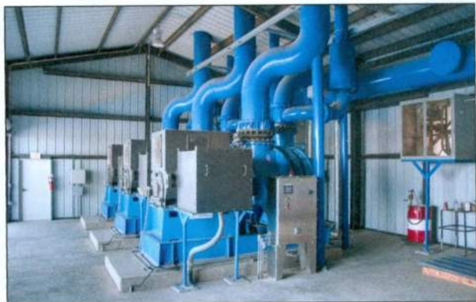
The Pine Bluff (Ark.) Wastewater Utility installed three new blowers at the Boyd Point Wastewater Treatment Plant to support its new fine-bubble aeration system.
